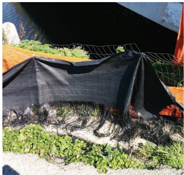
Wire mesh, silt fencing & orange plastic mesh deteriorating on site boundary, USA
