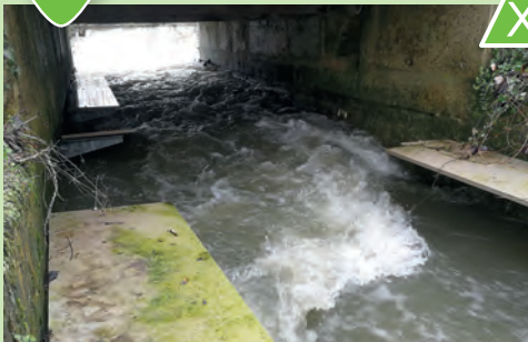
Mixed wood/concrete decking in 120 x 20mm thick slats is easily breakable and not recommended. Source: GREGE.
