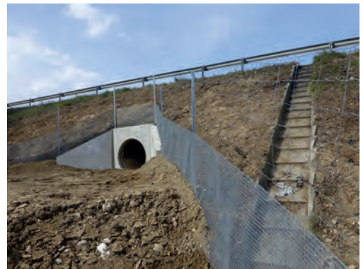
Small fauna passage at Velaux A7 motorway: view of the finalised device on the boring platform side. Source: Vinci Autoroutes/ASF network.
