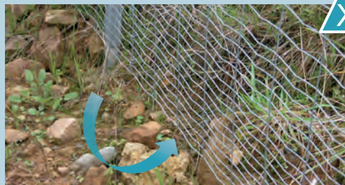
Unburied fence with progressive meshes, not pinned and leaving small fauna free access to the infrastructure coverage. Source: Cerema.
