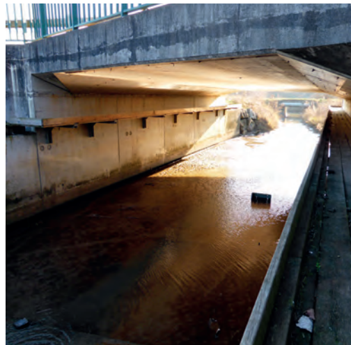
13 View of a wooden rail fixed to a corbelled bench. PNR Marais Poitevin. Source: Cerema.
