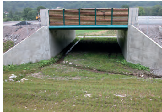
11 Underpass allowing the evacuation of run-off water towards the slope. Source: Cerema.
