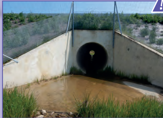
23 Flooded structure limiting the crossing of certain animals at least part of the year. Source: Cerema.
