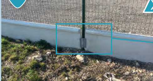
Treatment pond equipped with a concrete barrier with openings allowing free access to the pond by amphibians. RD 1004 (Bas-Rhin). Source: Cerema.
