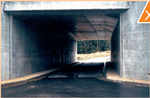
Example of a mixed fauna and forest restoration whose road has been surfaced and on which grass verges have been replaced by pavements.
