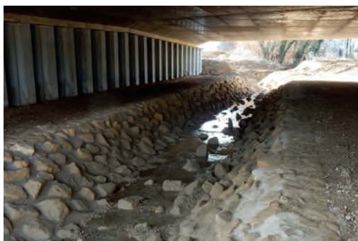
Restoration of a watercourse under the structure with masonry banks. Source: Cerema.
