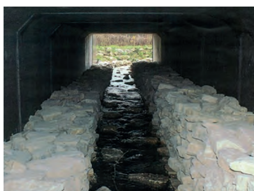
9 Development of a bench made of natural materials (sealed inside) in the crossing structure of the marten stream on RD12.
