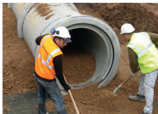
Manual implementation of a layer of soil inside a duct. Source: Vinci Autoroutes/ASF network.
