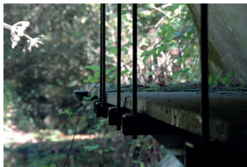
❸ Bench with 40cm wide by 50m long concrete decking and 60cm headroom. Cost: 6,000 € (installation under local authority control). RN164 (DIRO). Source: Cerema.
