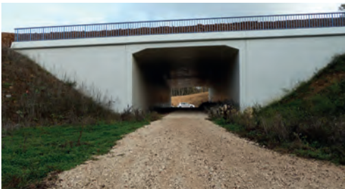
1 Agricultural and small fauna underpass. Source: Cerema.
