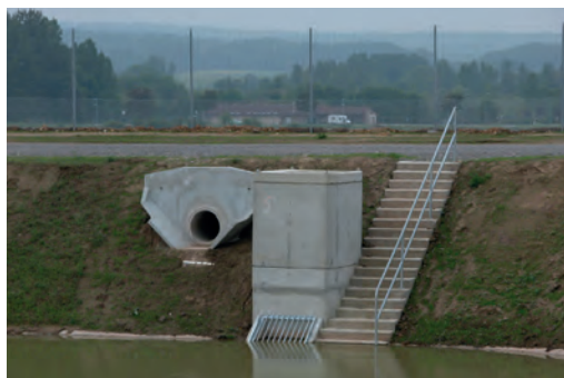
⑲ Treatment pond equipped with amphibian fences. Source: Cerema.
