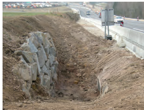
7 Access ramp protected by a masonry wall on the side of green rights-of-way. Source: Cerema.
