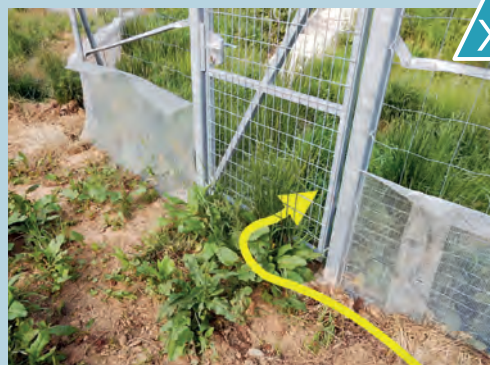
Broken fine mesh fence providing amphibians access to the coverage through the gate. Source: Cerema.
