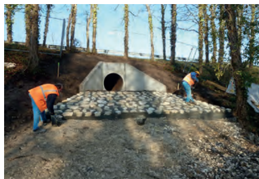
19 Construction of a masonry ramp before being covered with soil. Source: Vinci Autoroutes/ASF network.
