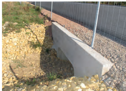
③ Funnel pit next to a small fauna passage of an infrastructure section located on the natural ground level. RD 16 (CD57). Source: Cerema.
