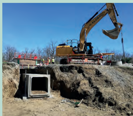
Implementation of elements of the structure. Source: TEC INFRA/Engineering office VRD & Project management
