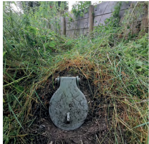
13 Check valve on downcomer preventing wildlife from accessing the coverage. Source: P. Fournier, GREGE.
