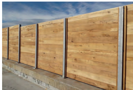
16 Screen of the La Buisse fauna passage (A48 – Réseau APRR), made in non-chemically treated locust tree. The wood was removed locally from motorway rights-of-way and processed nearby (sawing and panel manufacturing). In order to determine the strength class of this wood for sizing the panels, a selection of boards was subjected to bending tests. Source: APRR.
