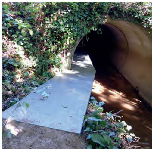
12 Example of a connection to the bank. Source: Cerema.
