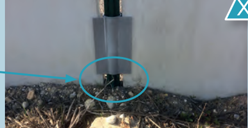
Opening in the device constituting an entry point. Source: Cerema.
