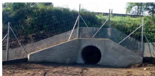
Amphibian fence bypassing the structure head. Source: Cerema.
