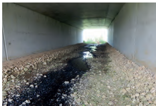
Example of a work in which some bends have been made in the low-water bed. Source: Cerema.
