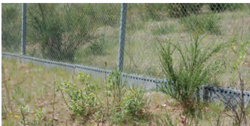
Edge in recycled plastic. B10 motorway, Germany. Source: Cerema.
