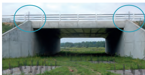
Return fence running along the walls and connected to the railing of the structure. Source: Cerema.
