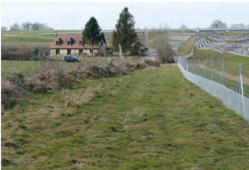
④ Construction of a swath on the edge of the A150 motorway. Source: OGE - Vincent Vignon.
