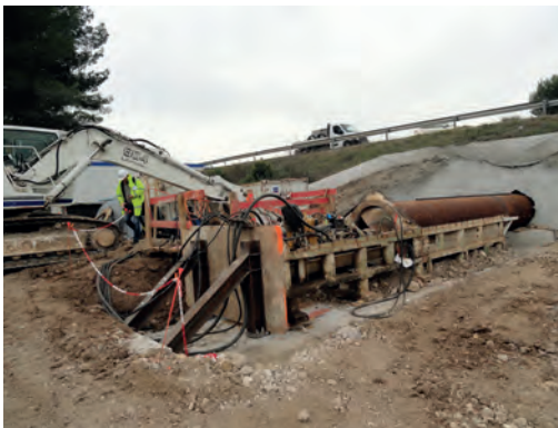
Small fauna passage at Velaux A7 motorway: View of the boring machinery. Source: Vinci Autoroutes/ASF network.
