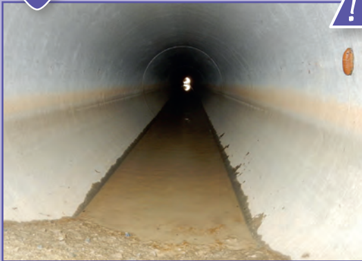
22 Build-up of materials at the outlet of the structure preventing drainage of the structure. Source: Cerema.
