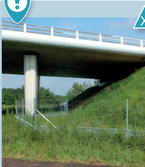
Poor connection of the fence that passes under the structure and reduces the space available to wildlife. Source: Cerema.
