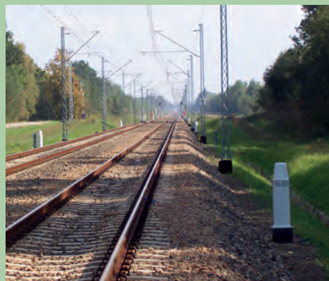
2 UOZ-1 post installed along a railway track.
