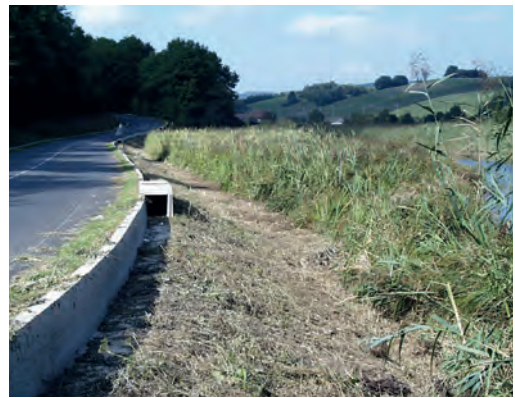
Maintenance of the amphibian passage of the Grand Lemps National Reserve. Source: Cerema Centre Est - V. Billon.
