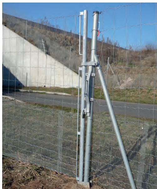
10 Correctly wired braced fence without a concrete threshold or bar or tensioning cable. Source: JBS Métallerie.
