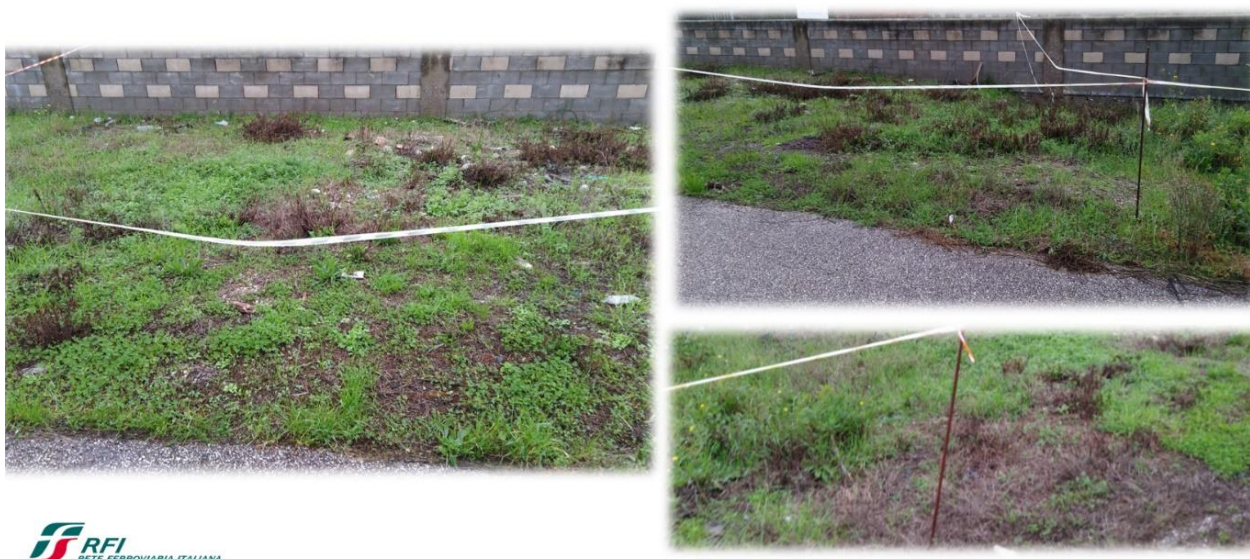
Figure 33: RFI - Hot Foam Method-3 - (e) results after 17-25 days from the application, (f) results after 45 days from the application
