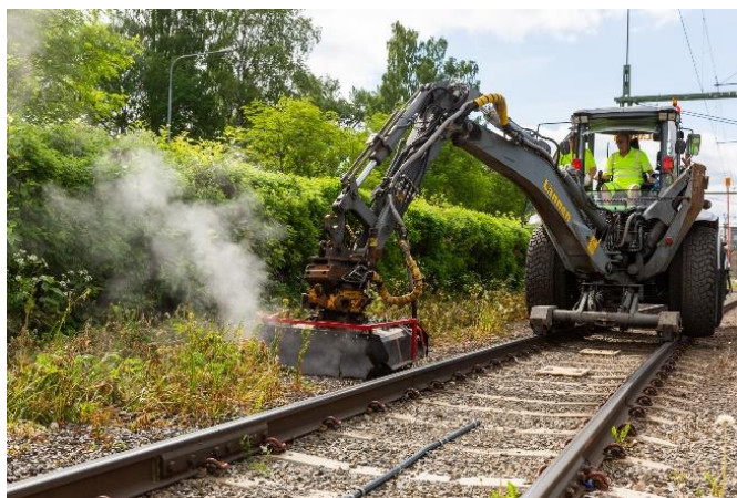
Figure 28: TRV - Hot Water - the equipment that was evaluated in Östersund
